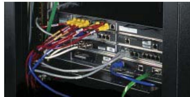
This Cisco 7200 Series router acts as the core gateway to Altera's corporate wide area network (WAN) and the Internet.
